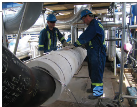
FIGURE 5. Shown here are two insulators installing single-layer calcium silicate pipe insulation at a petroleum refinery
