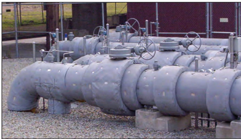
FIGURE 7. This photo shows several pipes completely insulated with removable and reusable insulation blankets made with coated-glass fiber fabrics. This type of insulation has the advantage of being able to be removed without damage to allow inspections and maintenance of the piping and equipment, then reinstalled with minimum extra labor
